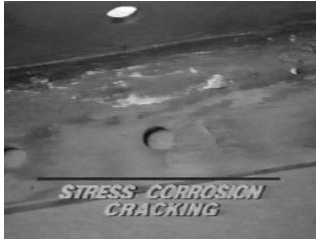
Figure 74. Stress corrosion cracking may be identified by the presence of multiple, fine cracks in high-strength alloys.
