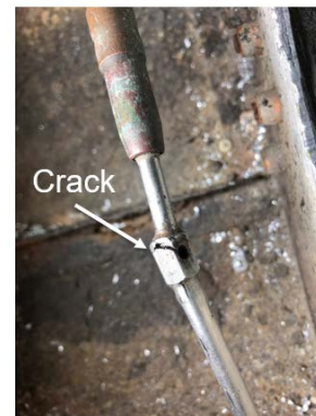
Not Severely Corroded
