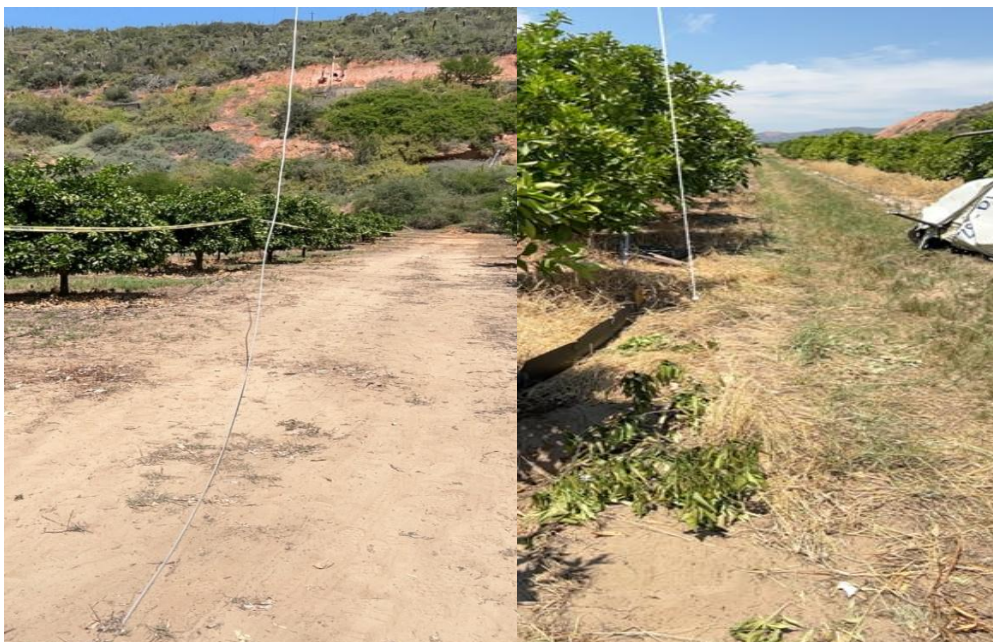
Figures 3 and 4: The damaged powerline after the accident.
