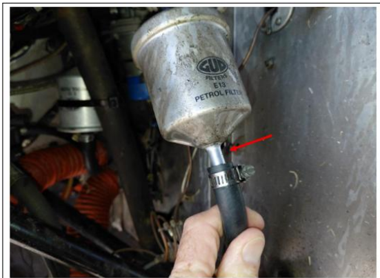
Figure 5: A loose inlet fuel pipeline on the left fuel filter.
