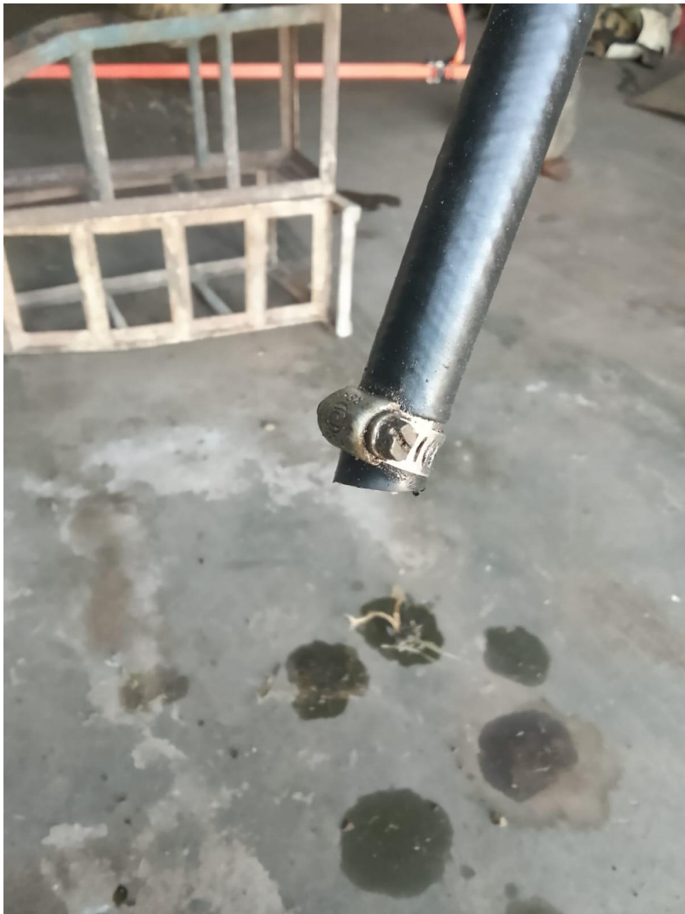
Figure 5: The affected clamp still attached to the hose.
