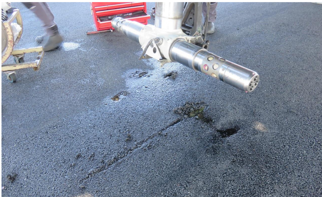
Figure 3: Damage caused to the runway surface where the aircraft had stopped.
