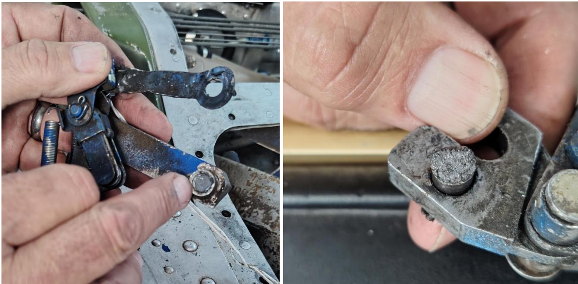
Figures 5 and 6: A closer view of the sheared down-lock support assembly pin.
